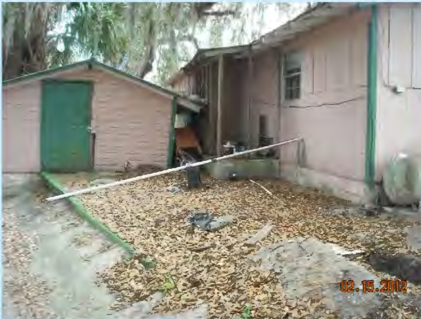
Washing machine discharge
