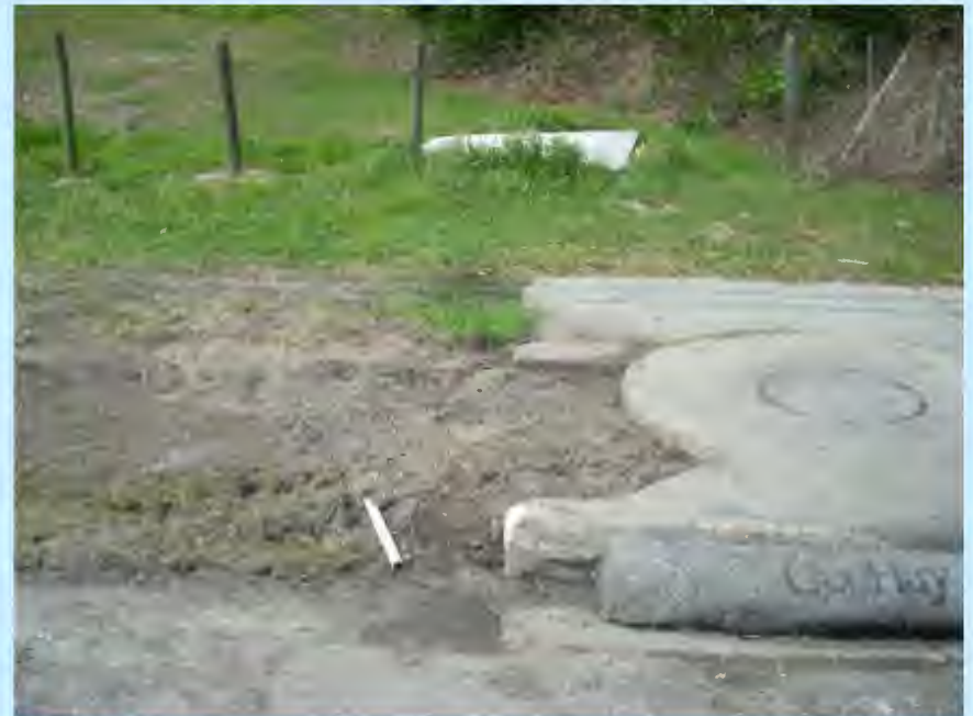
Unknown pipe to inlet
