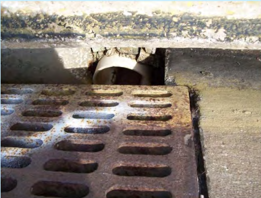
Unknown pipe into storm sewer inlet
