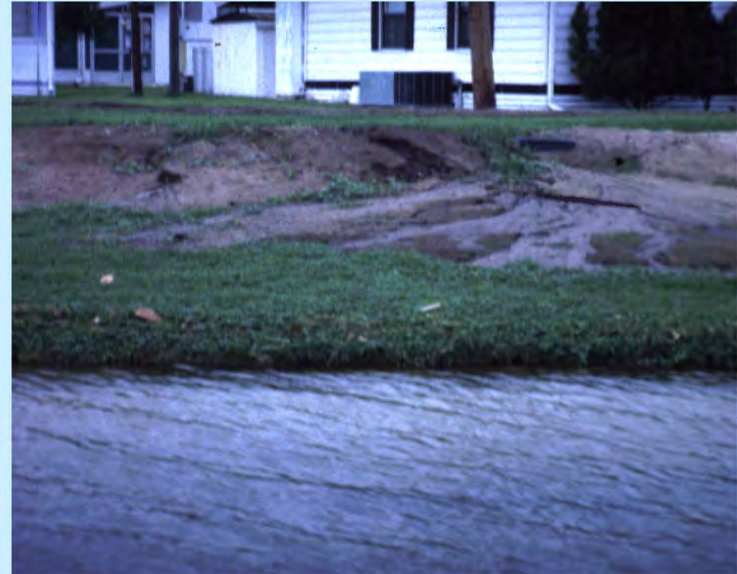
Failing septic tank
